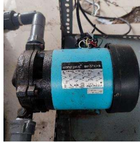
Gambar 3. 4 Booster Pump BR-371CPA
