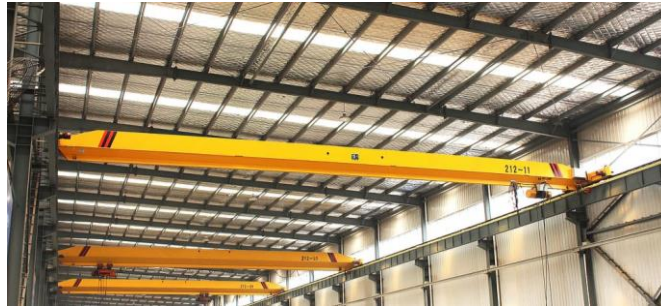
Gambar 3.4 Overhead Crane Single Girder
