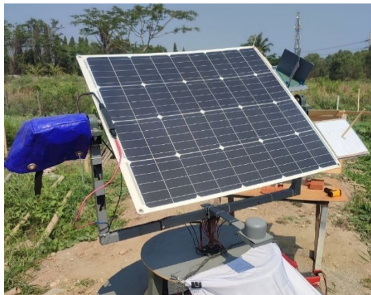
Gambar 4.3 Kondisi panel surya kegelapan shading 0%
