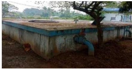
Gambar 3.3 Reservoir (Tandon Air)
