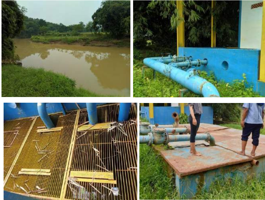
Gambar 1. Sumur Intake Sungai Cidurian
