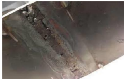
Gambar 2.3 Cacat Incomplete Fusion (Rizvia & Alib, 2019)
