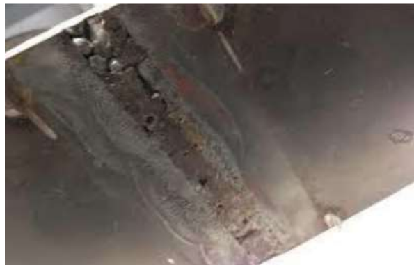
Gambar 2.3 Cacat Incomplete Fusion [7]
