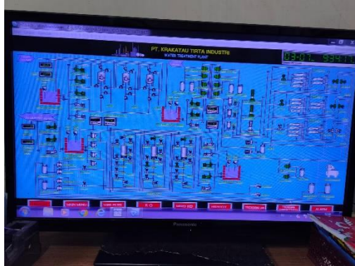
Gambar B.1 Control Panel Water Treatment Plant PT X
