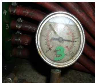
Gambar 4.4 Indikator tekanan air pompa cooling tower
