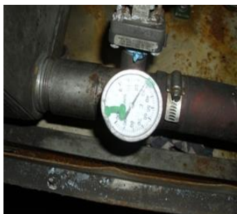
Gambar 4.2 Indikator temperatur air cooling tower input
