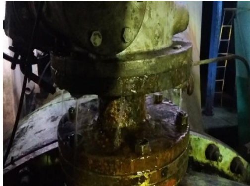
Gambar 4.5 kebocoran sealing cooling water
