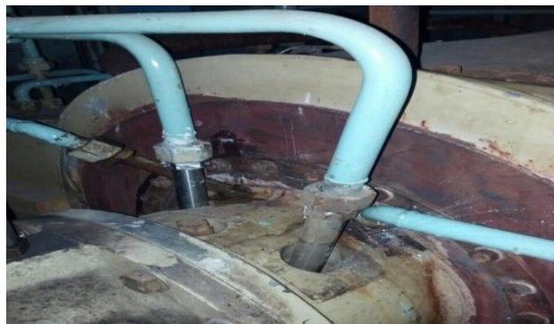
Gambar 4.8 Letak seal cooling sisi rear bearing
