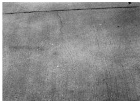
Gambar 3.18 Retak Susut ( Shrinkage Cracks )
