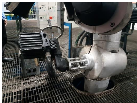
L3. Gate Valve MOV 30
