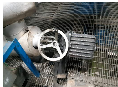
L4. Gate Valve MOV 30
