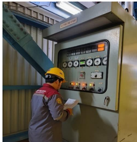
Gambar 5. 2 Control turbin startup board
