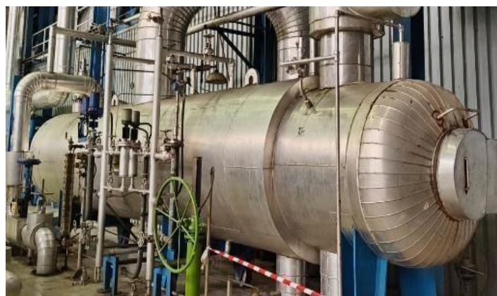
Gambar 3.11 High Pressure Heater
