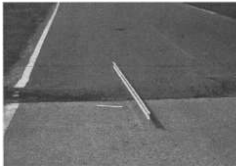
Gambar 3.19 kerusakan sungkur ( Shoving )
