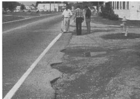
Gambar 3.10 cacat tepi perkerasan ( Edge Cracking )
