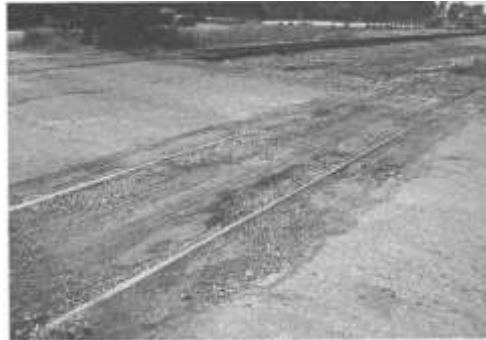
Gambar 3.17 kerusakan pelintasan jalan rel ( Railroad Crossing )
