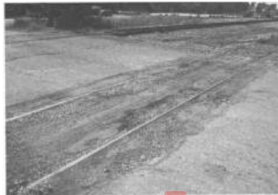
Gambar 3.17 kerusakan pelintasan jalan rel ( Railroad Crossing )
