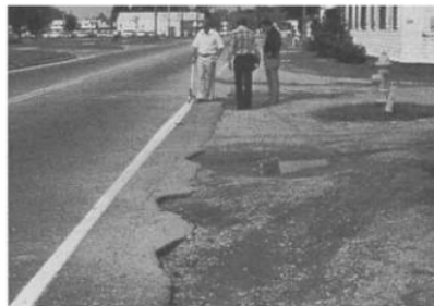
Gambar 3.10 cacat tepi perkerasan ( 23 Edge Cracking )
