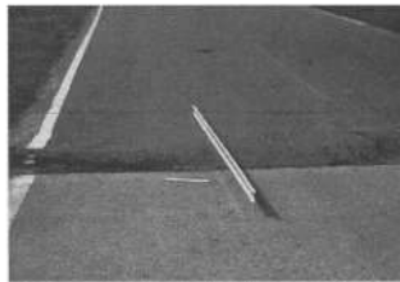
Gambar 3.19 kerusakan sungkur ( Shoving )
