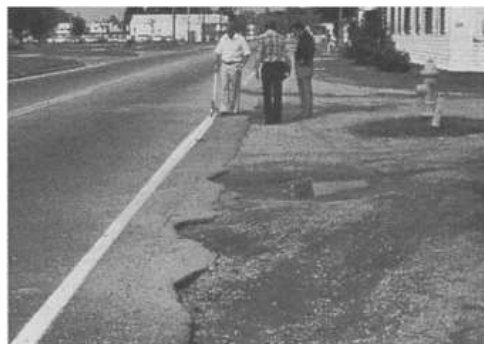
Gambar 3.10 cacat tepi perkerasan ( Edge Cracking )
