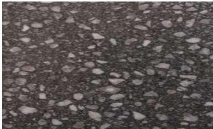
Gambar 3.17 Jenis Kerusakan Pengausan ( Polished Aggregate )
