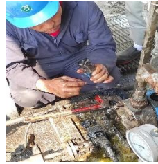
Gambar 4.14 Pembersihan Hydraulic Filter Oil
