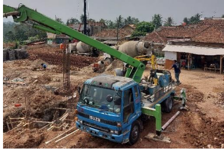
Gambar 4.5 Mobile Concrete Pump
