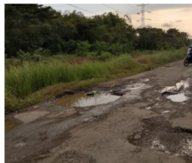
Fig.1 Masjid Priyayi road conditions.
