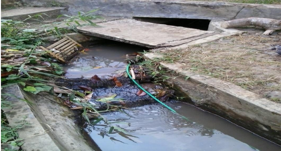
Figure 3 : Secondary II irrigation channels
